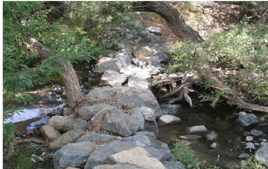
Grade stabilizer after installation and planting of riparian and wetland plants in spring of 2007.
